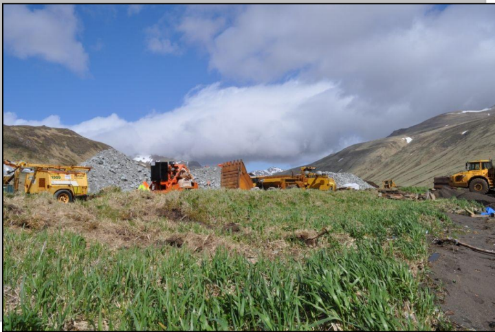
The project, located at the Head of the Bay, involves constructing two rock breakwaters, totaling about 1,500 feet.
