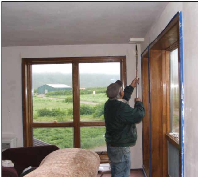
The Isanotski Corporation's B&B is being painted inside and out as part of a renovation project. Photo by Cindy Beamer.
