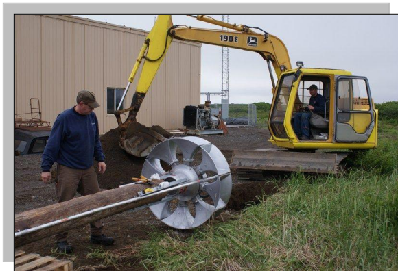
Cold Bay Public Works Director Shane Watson operates the excavator, while Mark Tans of Integrated Notification Systems looks on. Photo by Monty Martin.
