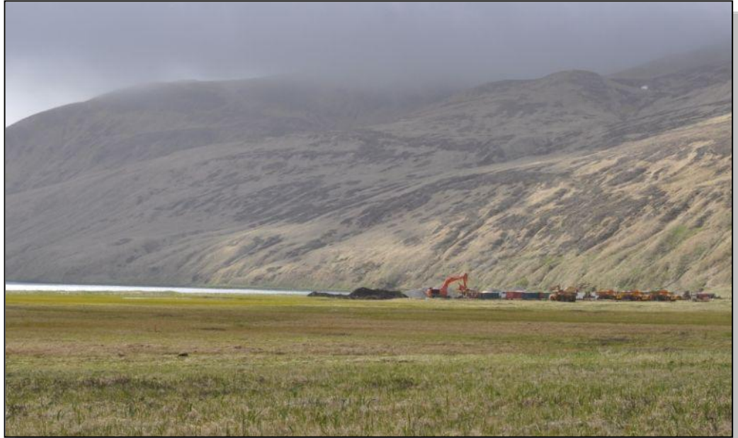
The new harbor is expected to provide space to 30 vessels, from 110 feet to 155 feet in length, in addition to smaller vessels. Photo courtesy: Mead & Hunt, Inc.
